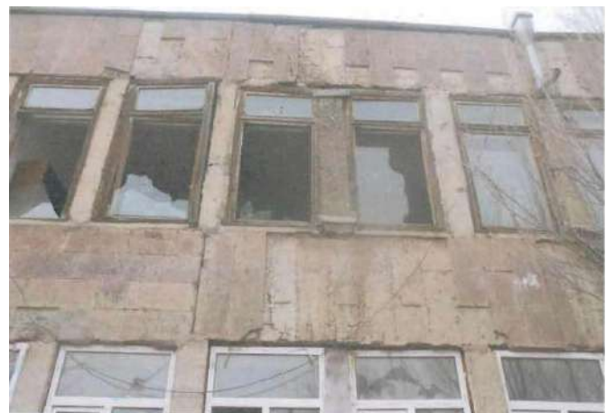
Picture 7. The exterior walls of the building are damaged, windows are broken, and the building is in a deplorable condition. Adjacent to the building there is some self-growing vegetation, which, being located close to the walls, undermines the foundations of the building and may be subject to removal.
